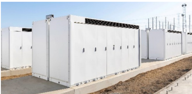
Sample imagery of a BESS enclosure
