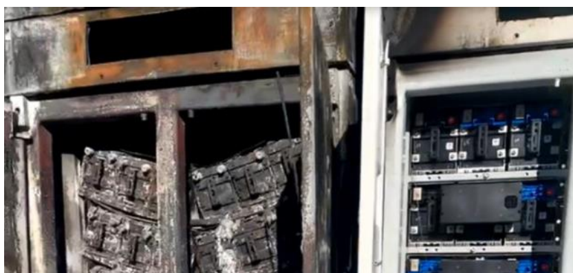
Figure 33: Charring to case and safe batteries to battery units adjacent to fire unit.
